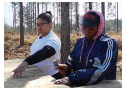
VSU students Briana Peebles (L) and Lillian Coffey assist with building a house for Habitat for Humanity in Lucedale, MS as part of VSU's 2013 Alternative Spring Break.
